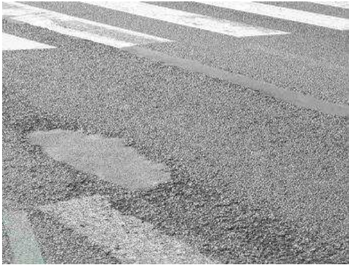
Figure C5 Delamination, fretting and ravelling
