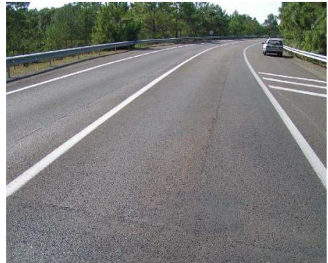
Figure C9 Poor transversal joint
