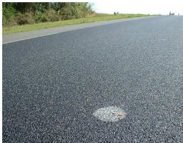
Figure C4 Satisfactory UTLAC – homogeneous texture
