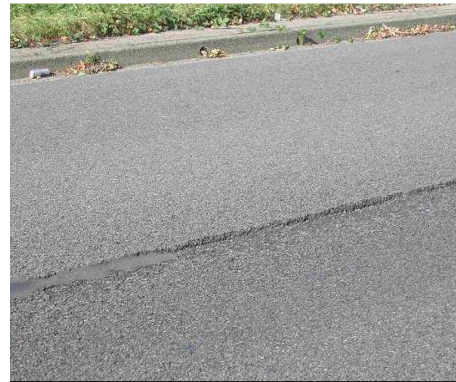
Figure C7 Ravelling on longitudinal joint
