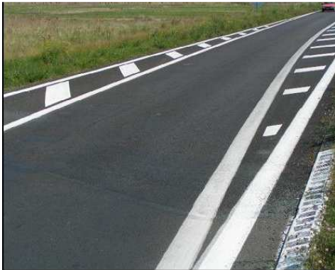
Figure C8 Transverse bump and localised fretting
